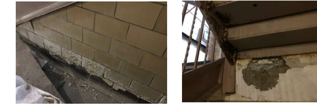
PICTURE A - STAIR 200 FIRST FLOOR PICTURE B - STAIR 200 INTERMEDIATE LANDING AT ENTRY
